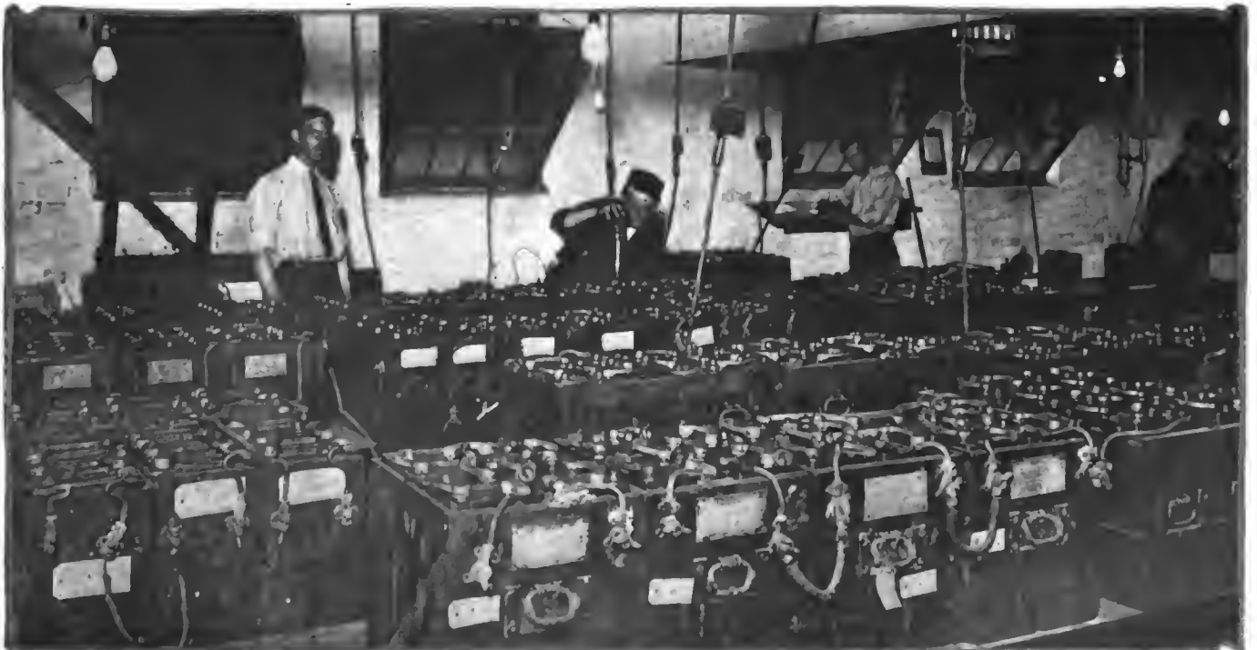
Battery room in the factory of the Baker Motor Vehicle Co., Cleveland, O.
